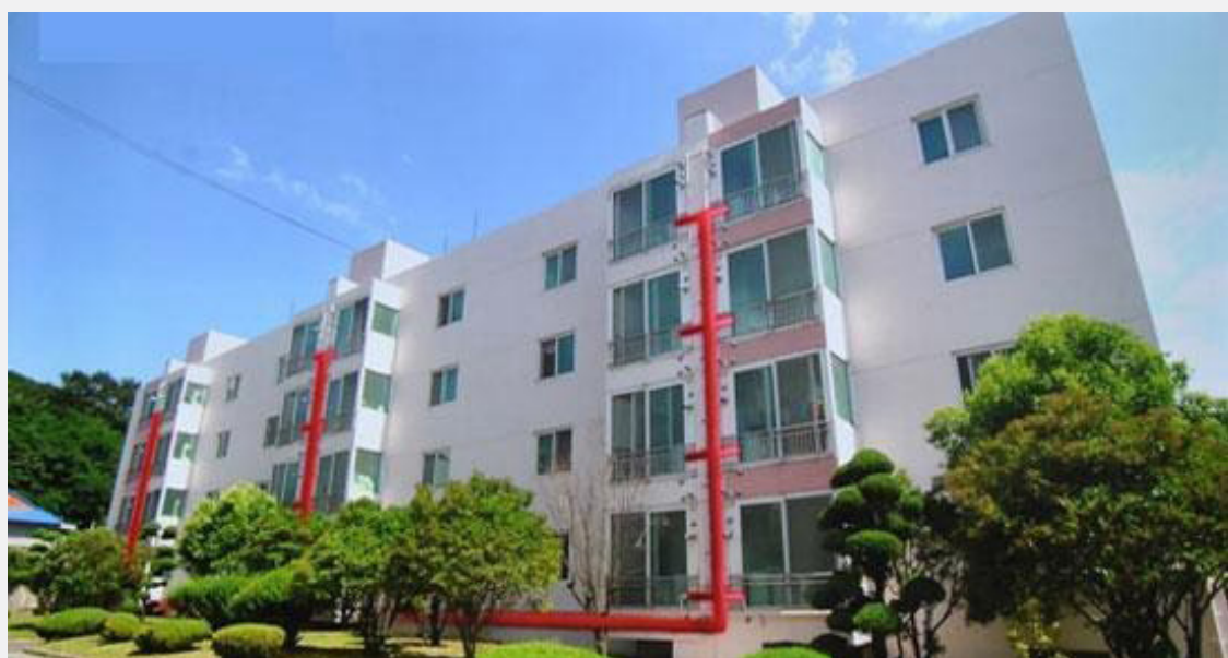
Figure 50 Hydrogen pipelines (red) installed on the external wall of the apartment (Shin, 2014)
